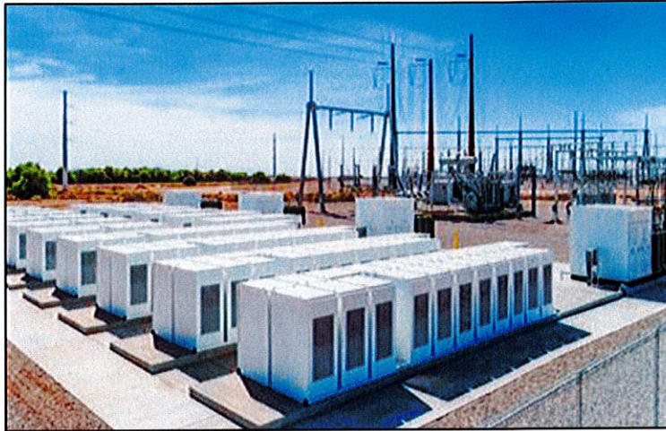
Figure 2b. Example self-contained energy storage system cabinet.
