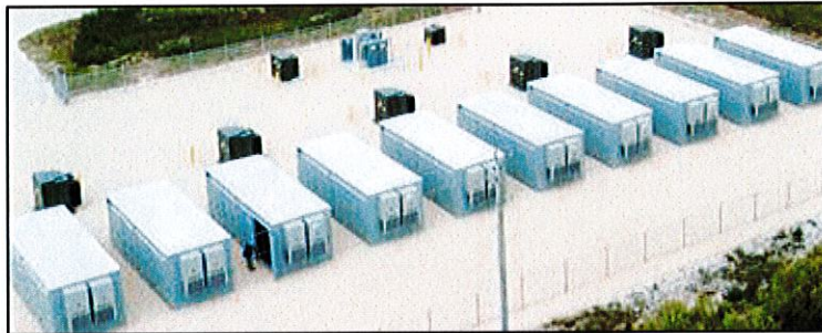
Figure 2c. Example self-contained energy storage system cabinet.
