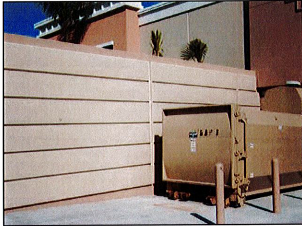
Figure 3a. Example of sound barrier (IAC Acoustics 2023).
